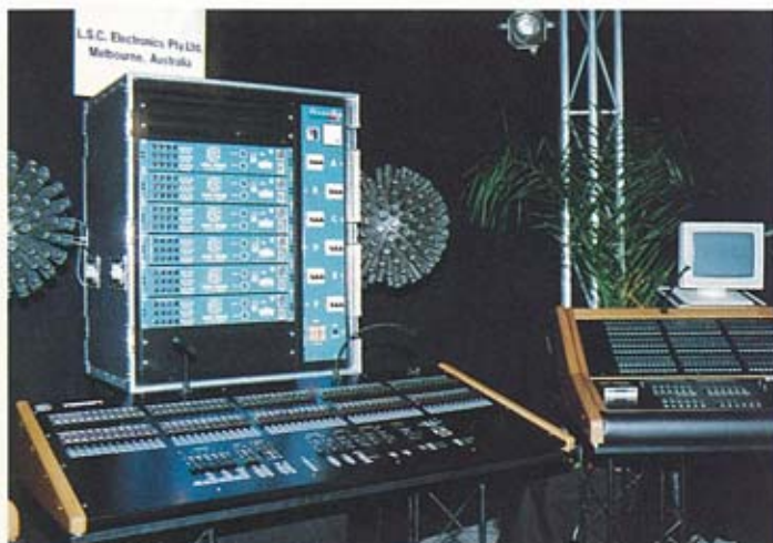
Part of the LSC control system line-up.
